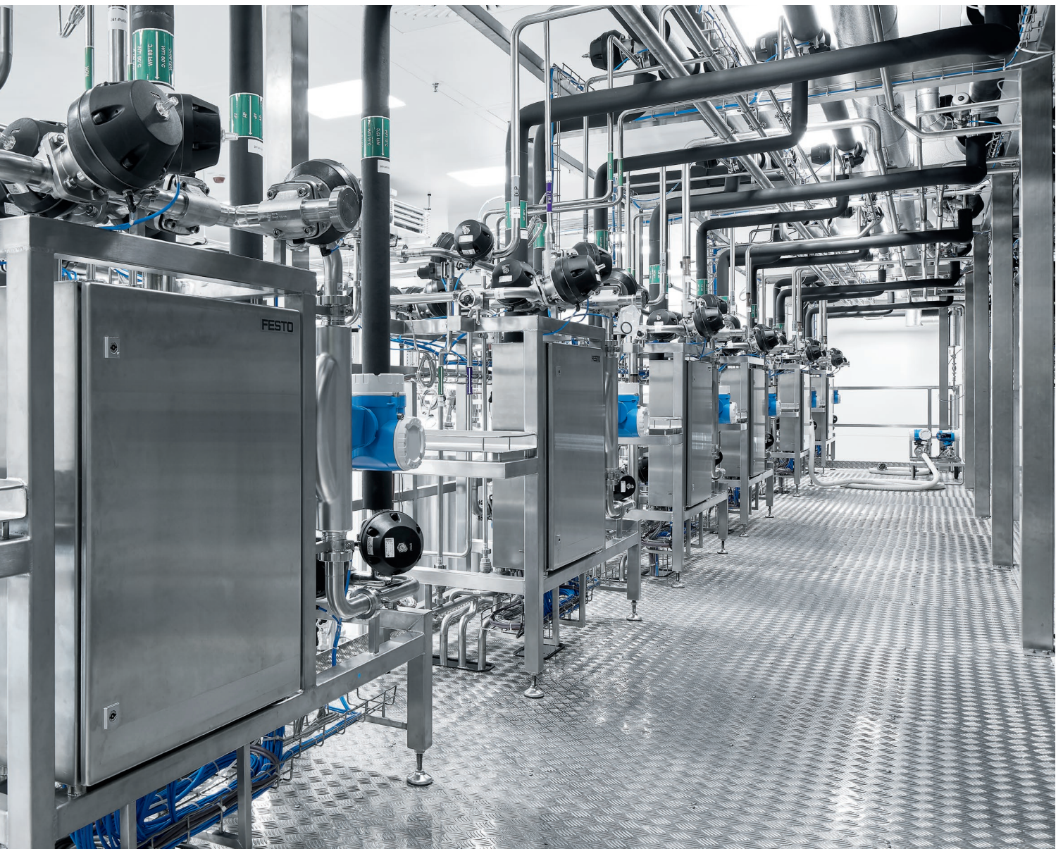
Incorporated as early as the planning stage: 6,000 components and 250 control cabinets from Festo.
